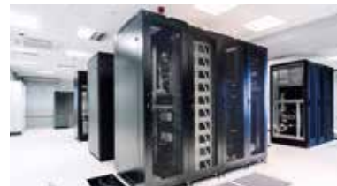
Connection of generators for a server room UPS (New Zealand). Series TH405.
