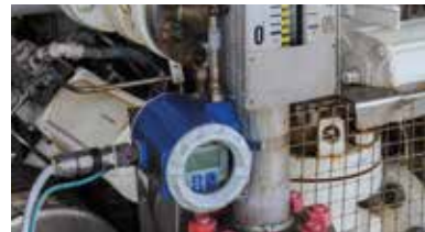
Connection of liquid level sensors (Shanghai, China). Series TH451.
